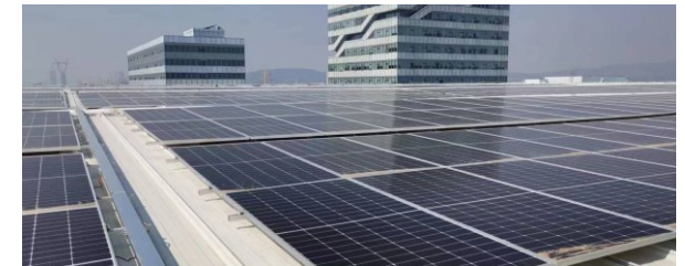
Photovoltaic Rooftop at the Headquarters Park
