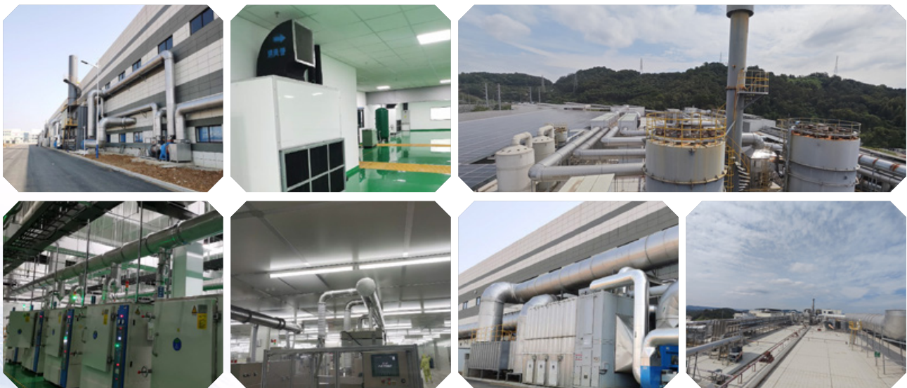
Exhaust Air Treatment Facilities 廢氣處理設施
