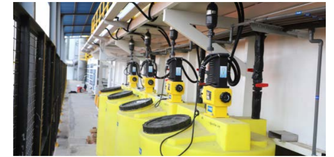
Facilities of the plant's wastewater treatment station
