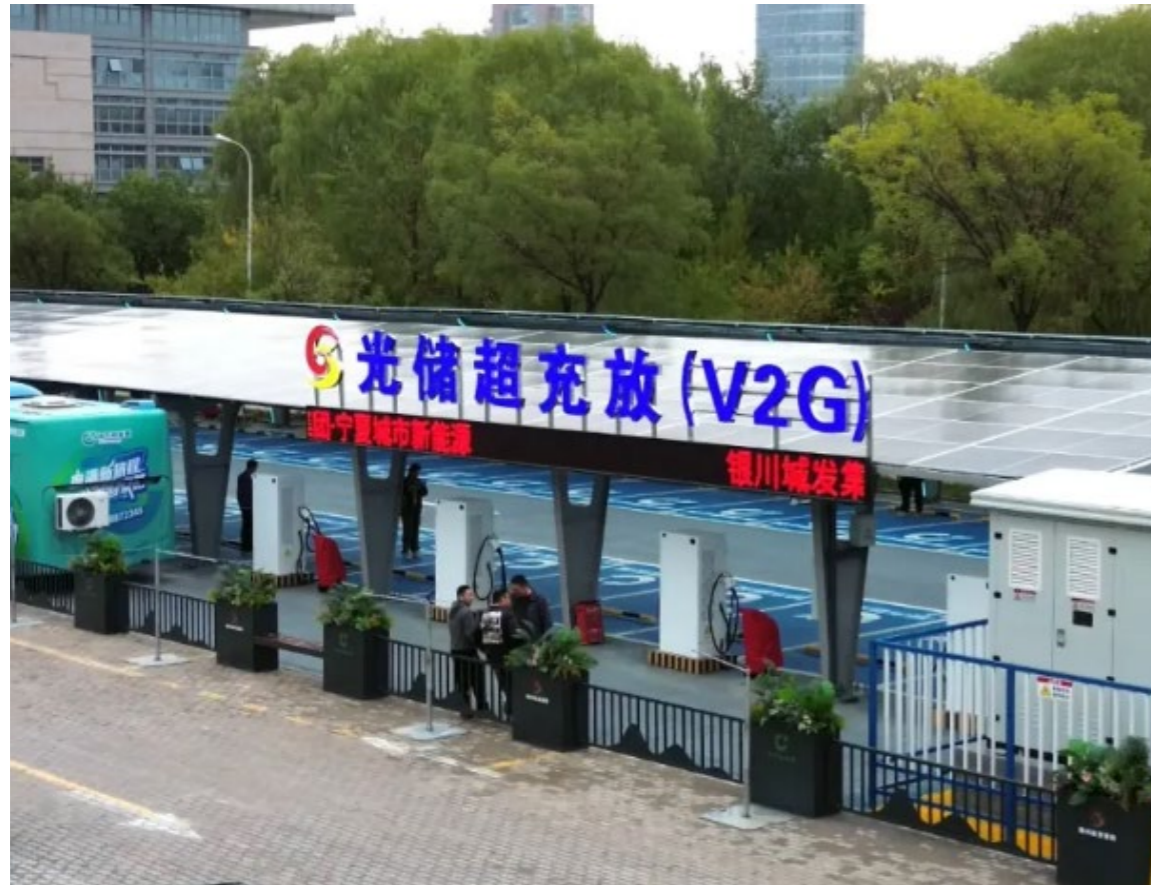
Uniview engages in building Ningxia Photovoltaic-Storage-Charging-Discharging Demo Station
