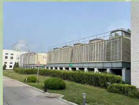
The cooling towers improve heat exchange efficiency and reduce water consumption 冷卻水塔優化換熱效率，降低用水量
