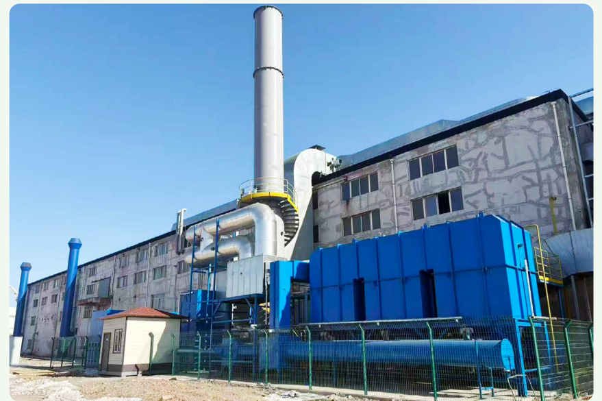
Upgrading of Waste Gas Treatment Equipment in the Coating Workshop at Panjin Facility
