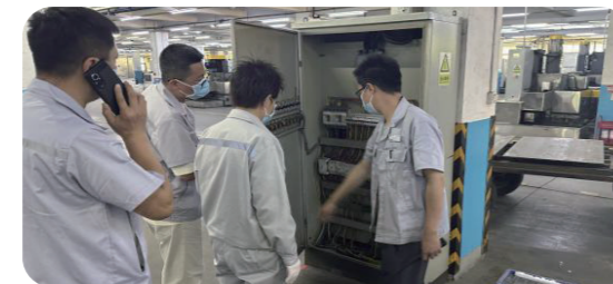
On-site Safety Hazard Investigation
