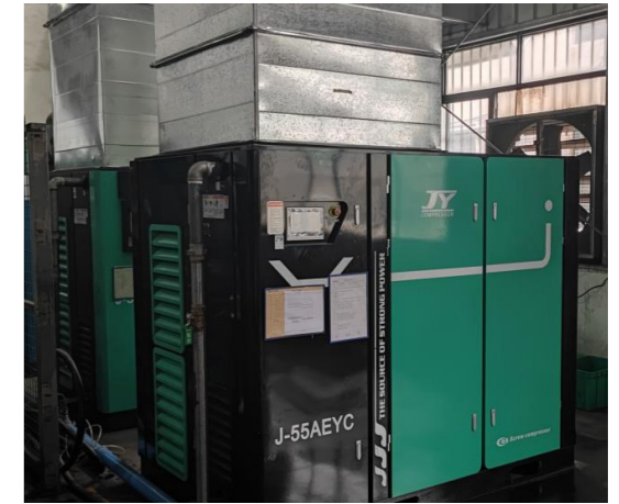
Air Compressor System
