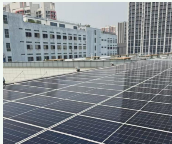
Rooftop Photovoltaic Panels at the SACA's Facility
