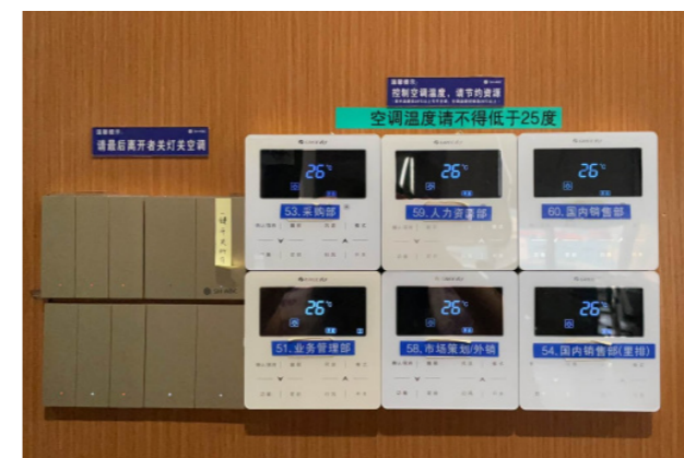
Posted Reminders for Air Conditioning Management
