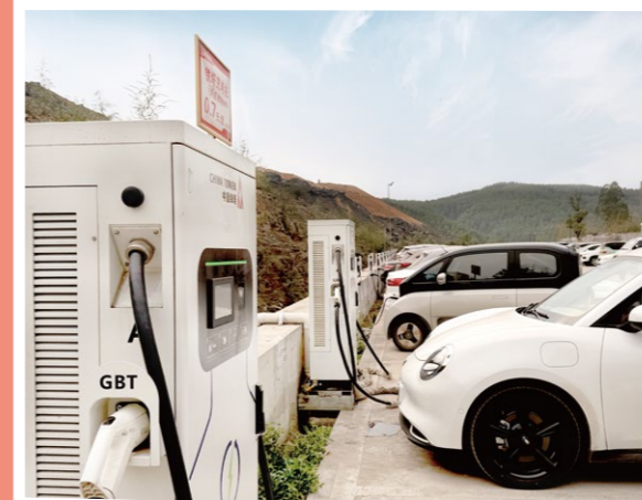
Electric Vehicle Charging Facilities
