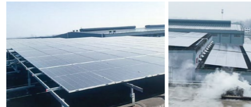
Photovoltaic Power Generation
