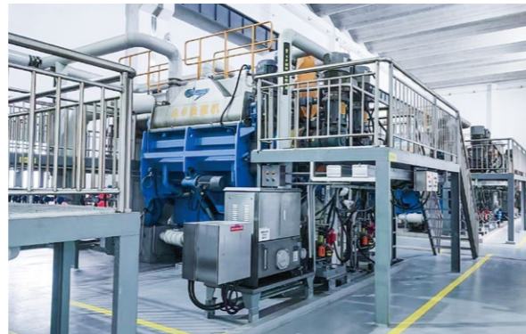
Pulping white water recovery equipment
