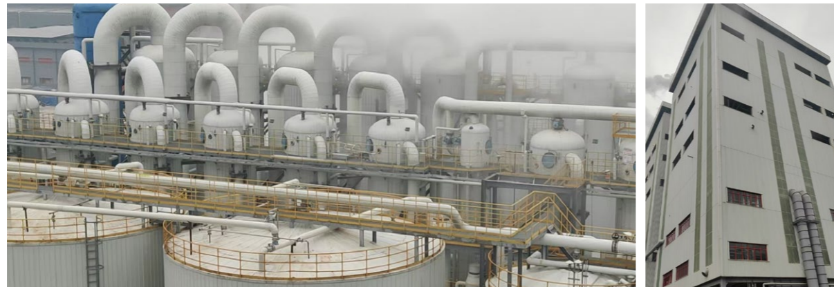
Black Liquor Alkali Recovery and Waste Heat Utilization System
