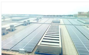
Photovoltaic Project Facilities at the Base
