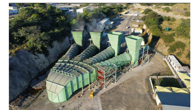
Completed surface ventilation shaft fans.
