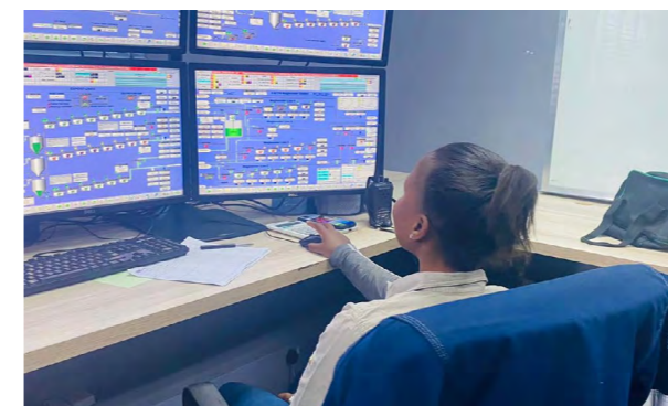
The magnetite technology team purchased multiple monitoring screens for the new process control room, upgrading the equipment for the process control facility.
