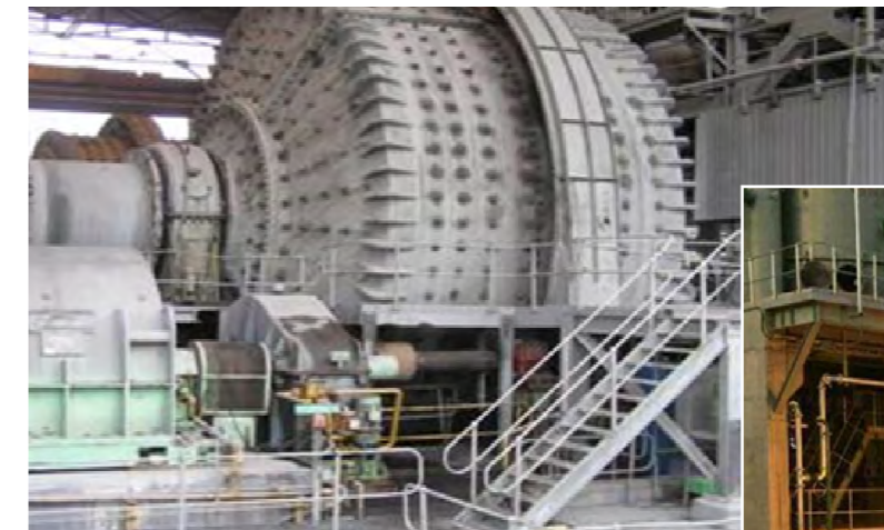
Autogenous Mill Unit in Concentrator
