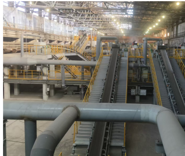
钢渣磁选加工生产线 The steel slag magnetic separation processing line
