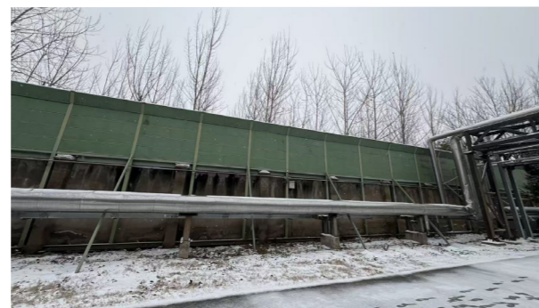
Noise Barrier Installed between Gujing Plant and Residential Area to the East of the Company
