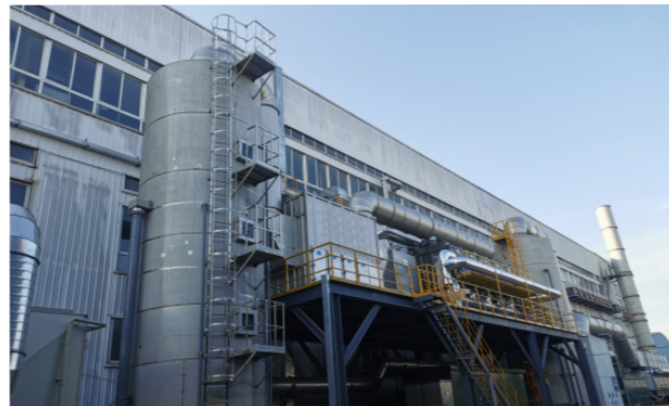
Air emission treatment facility
