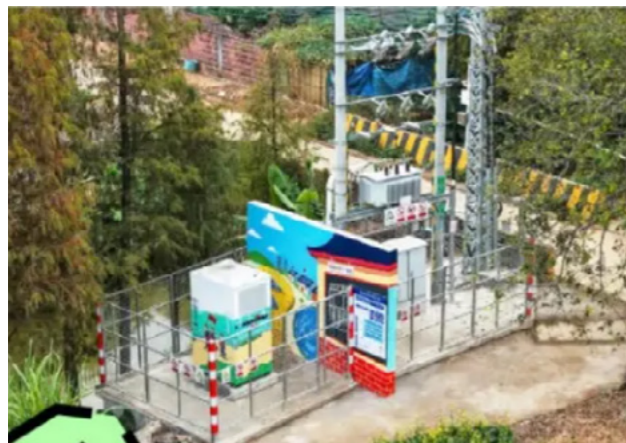
Haishou Island Multi-Microgrid Project, Guangdong Province
