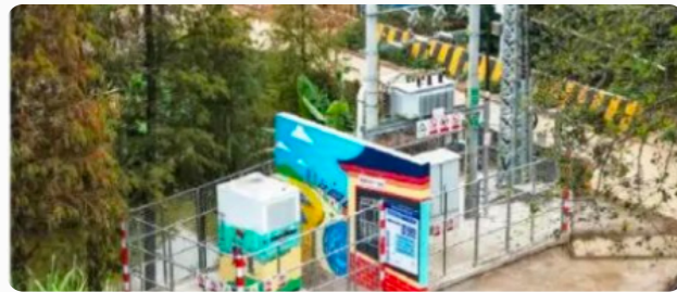
Foshan, First Distribution Area Energy Storage System officially connected to grid and put into operation at Haishou Island Project
