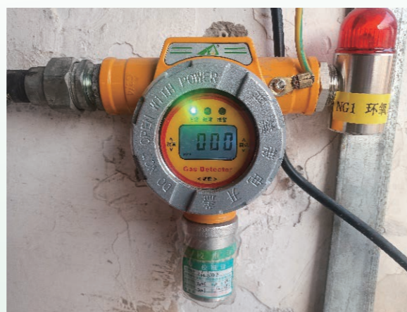
Toxic gas alarm
