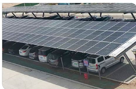
Solar power generation
