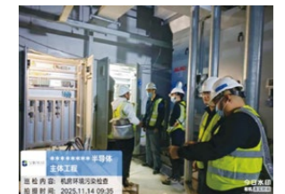
▲ Inspection of Environmental Pollution in Machine Rooms
