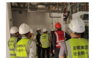
▲ Investigation and Treatment of Leakage Hazards in the Chemical Area
