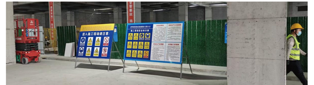
▲ Safety Warning Signs and Markings
