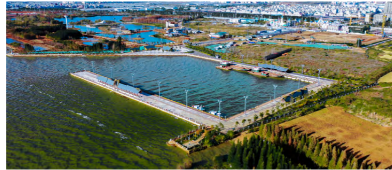
云南昆明呈贡新城码头项目创新实施“零废水入湖”方案 The Chenggong New City Wharf Project in Kunming, Yunnan, innovatively implements a "zero wastewater discharge into the lake" solution
