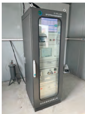
VOC online monitoring system VOC在線監測系統
