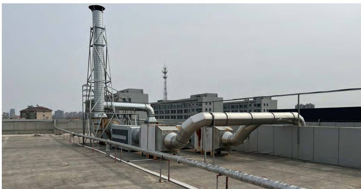
Activated carbon and photo-oxygen catalytic treatment equipment
