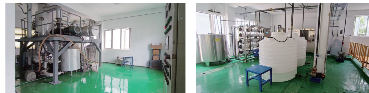
Reclaimed Water Treatment Plant
