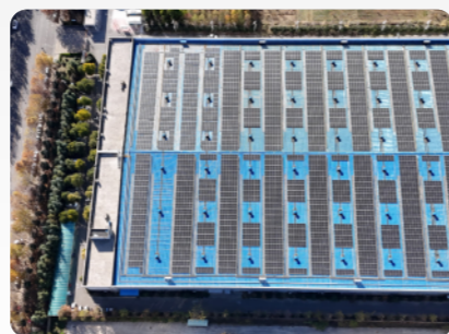
Factory Area Photovoltaic System
