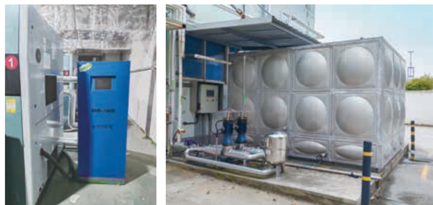
"Residual Heat Recovery" Facilities
