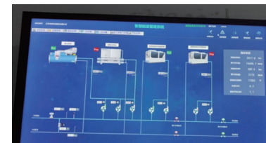
Intelligent and Efficient Central Air Conditioning System
