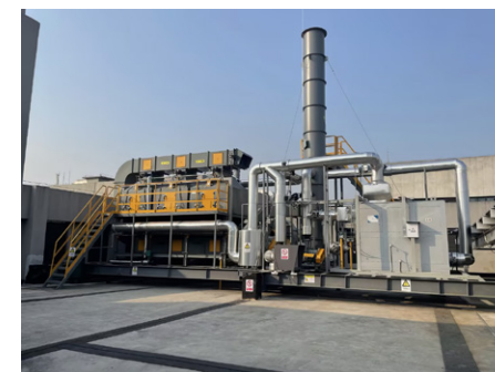
Waste Gas Treatment Facility
