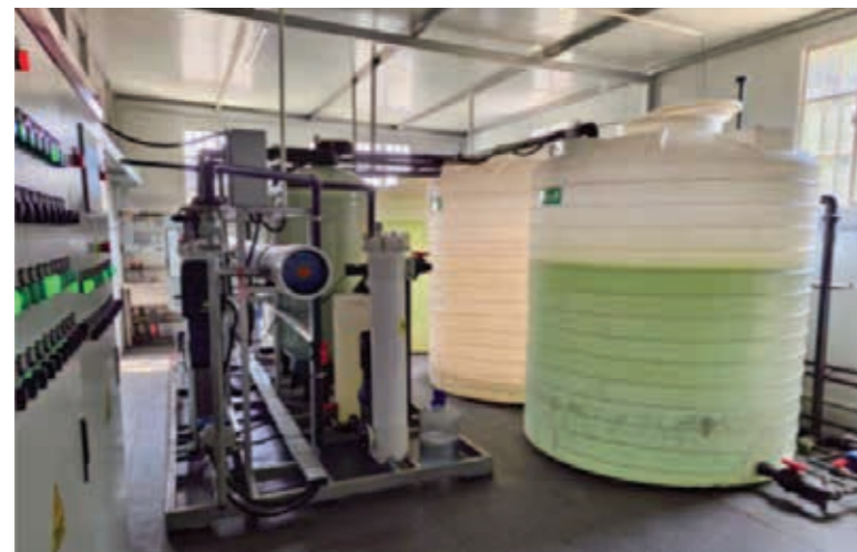
"Reclaimed Water Reuse" Facilities
