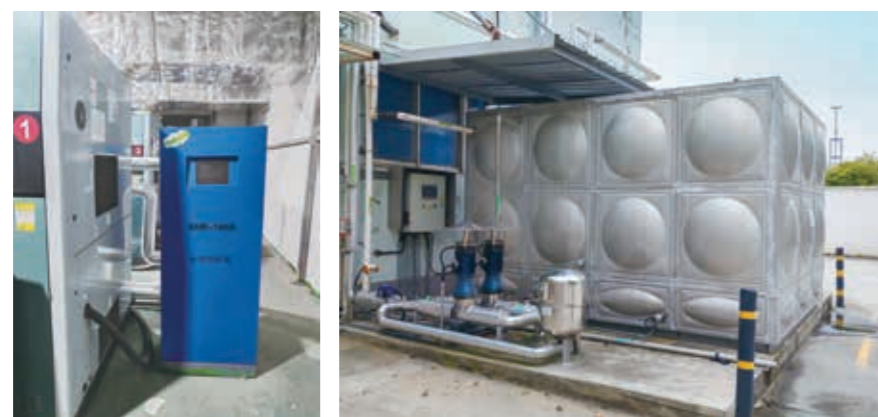
"Residual Heat Recovery" Facilities
