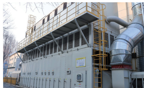
"Rotary Concentrator + Regenerative Thermal Oxidizer" Integrated Unit
