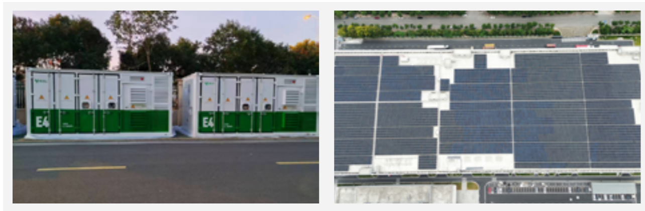
▲ Longshan Base II Power Storage Facilities
