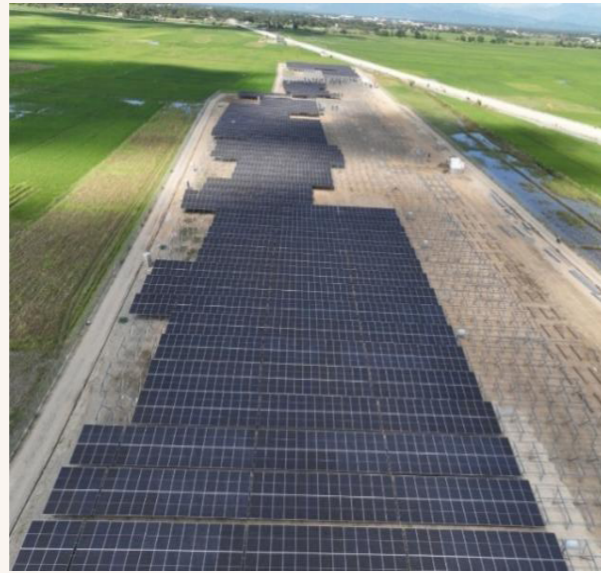
Site view of the 8.625MW project in the Philippines
