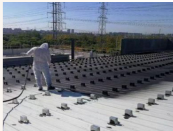
Nano coating roof photovoltaic
