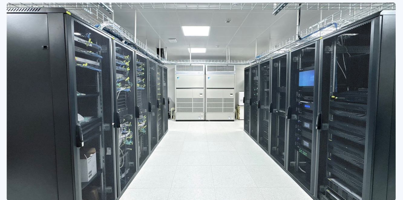
Marubi Building Computer Room
