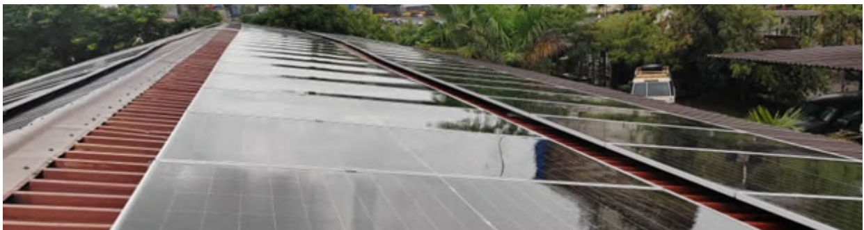
Ruashi礦場太陽能安裝工程 Solar Energy Installation Works at Ruashi Mine
