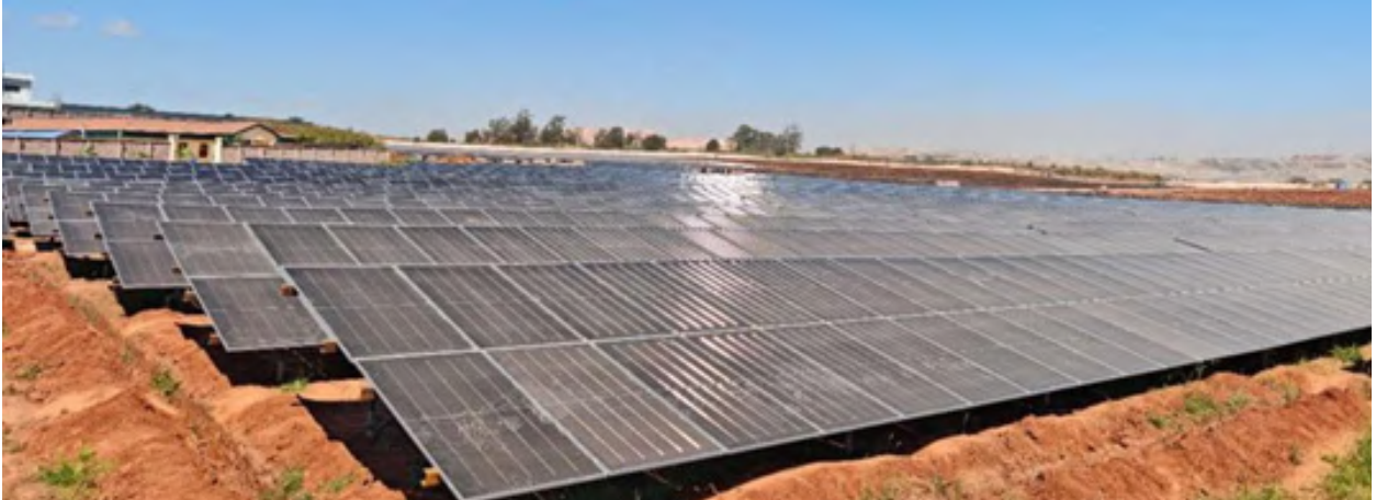
Musonoi 礦場光伏發電現場 Musonoi Mine Photovoltaic Power Generation Site
