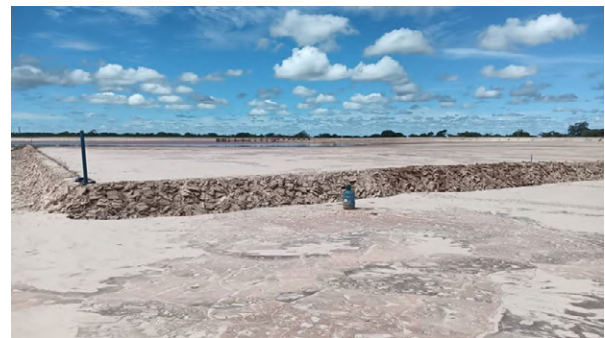
Kinsenda礦場在尾礦壩內設計建造「排水泥壩」 Kinsenda Mine designs and builds 'drainage mud dam' within the tailings dam
