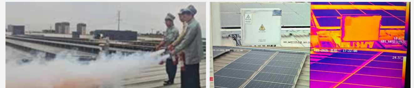
Rooftop Photovoltaic Fire Safety Management
