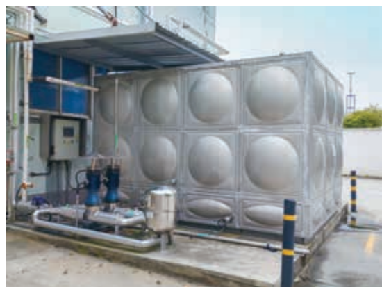
“餘熱回收”設施
