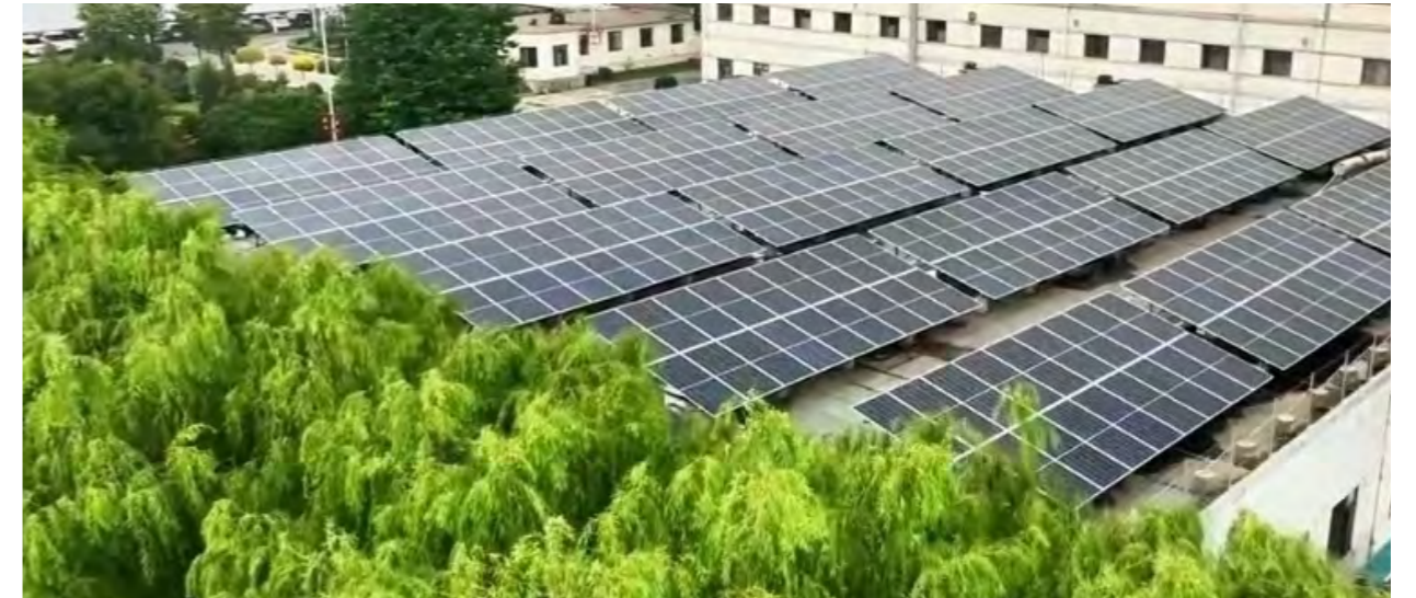
5.96 MW Distributed Solar PV Plant
