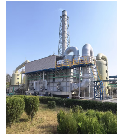
Waste Gas Incineration System
