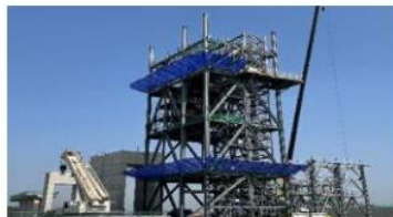
Figure 4: Acid Roasting Pre-Heater
