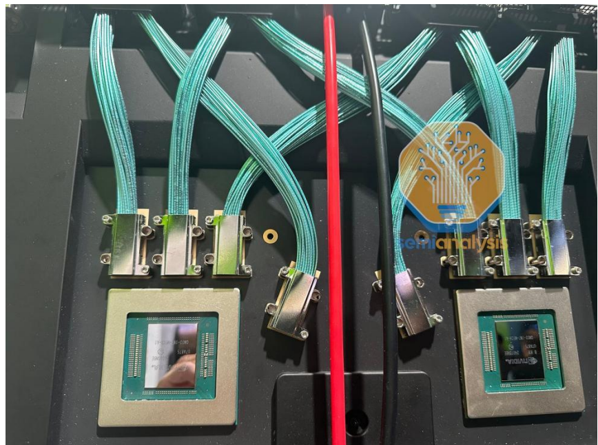
图 7: NVSwitch With 288 Copper Cables Per Switch
